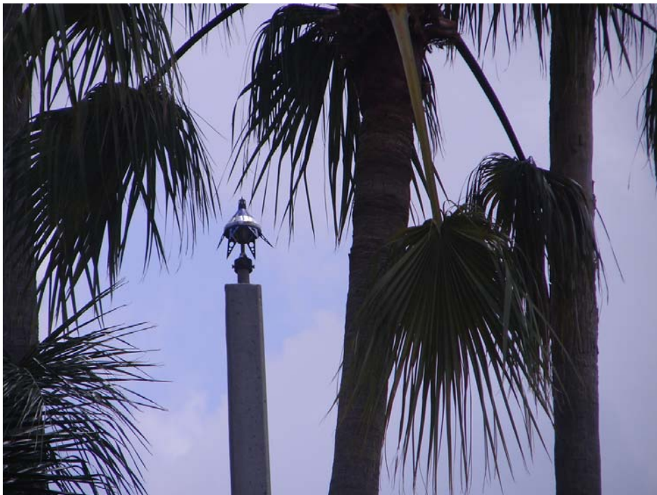
Fig. 6b: Close-up photograph of the Preactron 2 Millennium S 6.60 lightning rod mounted on top of an approximately 15 m high concrete pole.
